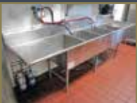
(17) S/S 2, 3, & 4-COMPARTMENT SINKS
